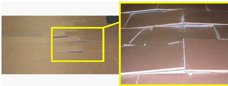
Figure 2: Tile separation from the sub-base in a radiant heat floor [Cocchetti, Comi, and Perego (2011)]
